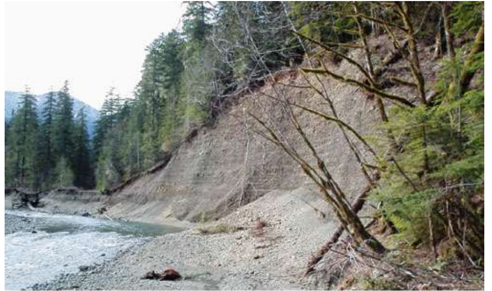
Main Dosewallips road washout from the east. The river now flows where the road once was.
