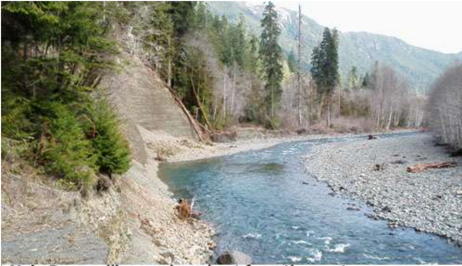
Main Dosewallips road washout from the west. The Forest Service's "instream" reconstruction alternative would build a road directly through the river here.
