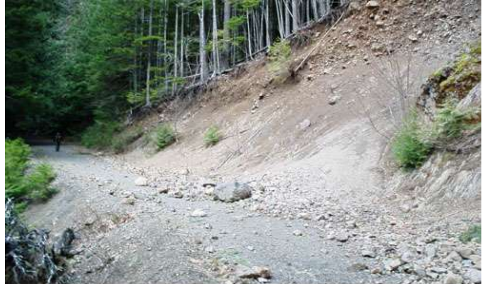
Eroding cut above Dose road.
