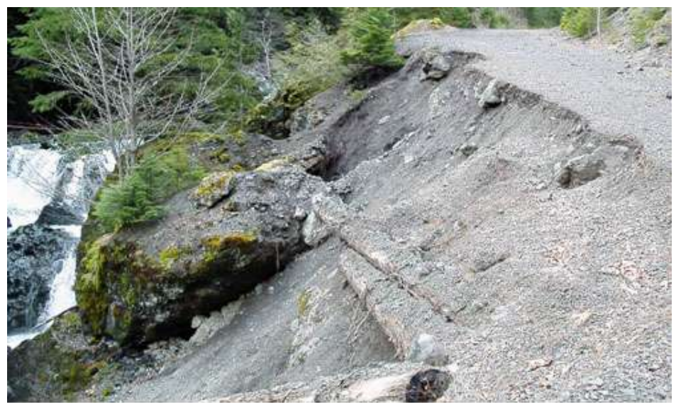
Road washout eroding into Dosewallips Falls in national park.
