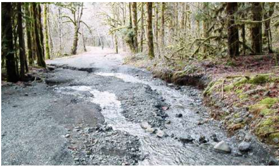
"Problem" Creek across Dosewallips road, one mile prior to the big washout.
