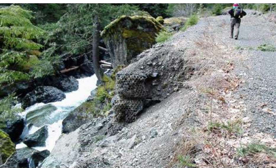
Failing gabions (wire cages of rock) above Dosewallips Falls.
