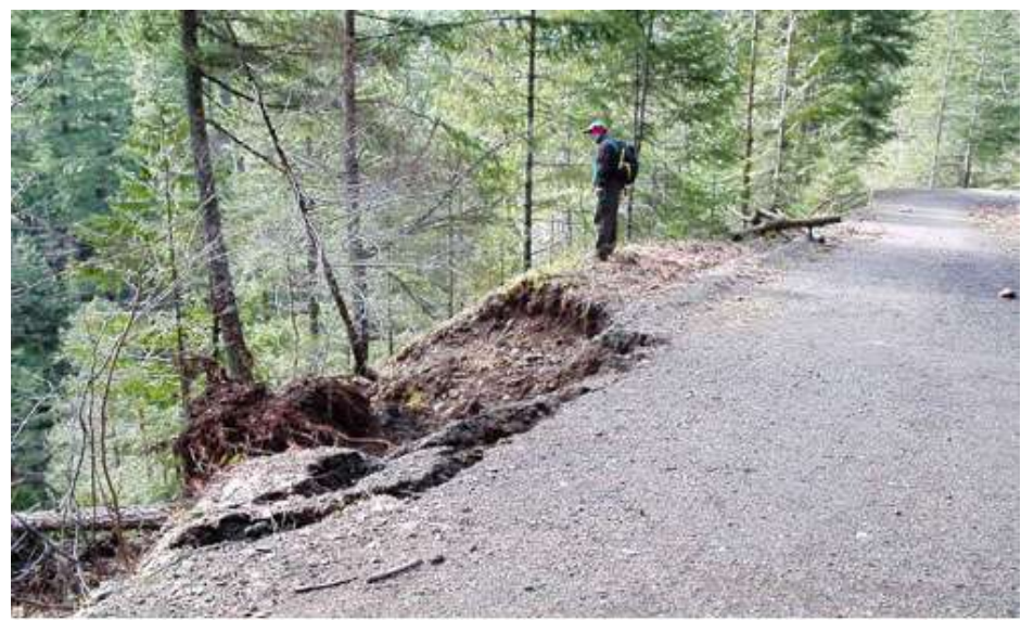
Road failure above Dosewallips River.
