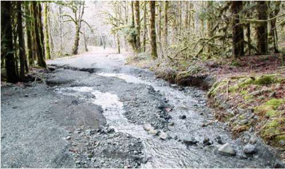
"Problem" Creek across Dosewallips road, one mile prior to the big washout.
