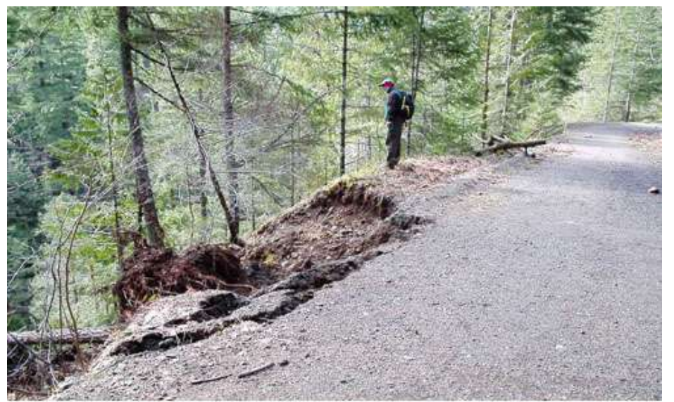
Road failure above Dosewallips River.
