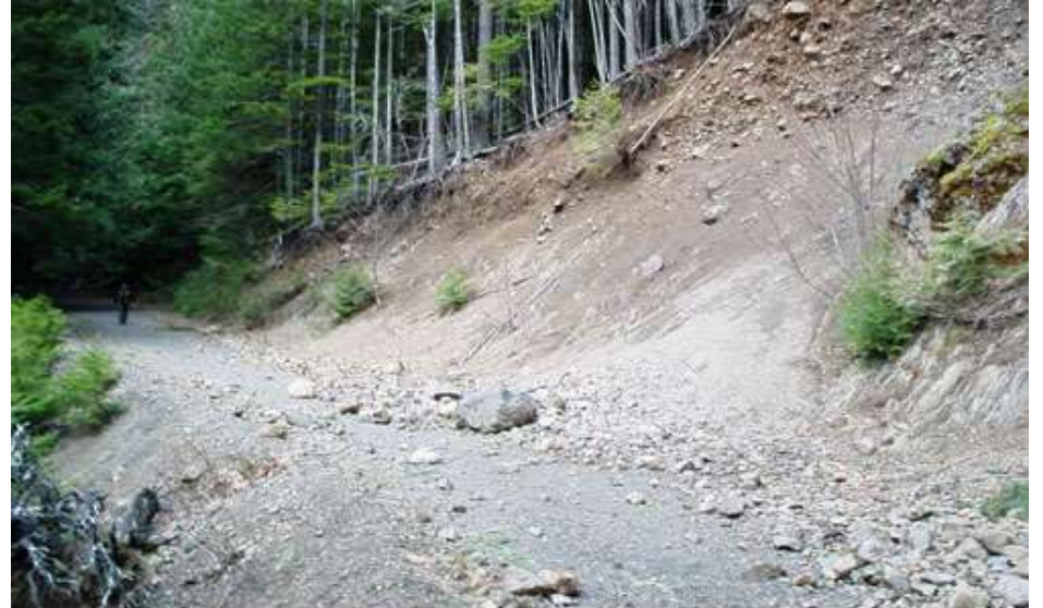
Eroding cut above Dose road.
