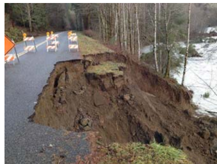
During this past December's storms, Dosewallips Road, mile 3, washed out again. At the time photo was taken, portions of the road were still sliding into the river. photo by Sallie Harrison
