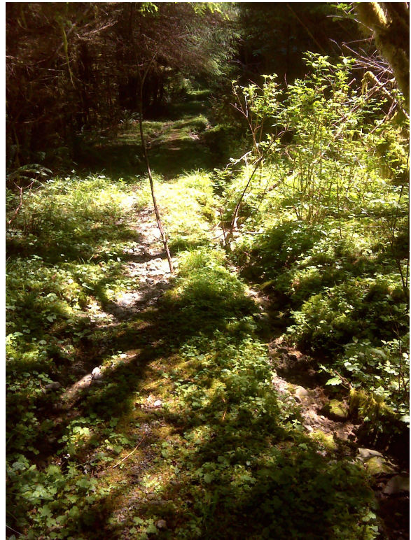
Photo # 2 2180200B N47 36.397 W123 57.588 Notes: gullying and erosion down edge of roadbed
