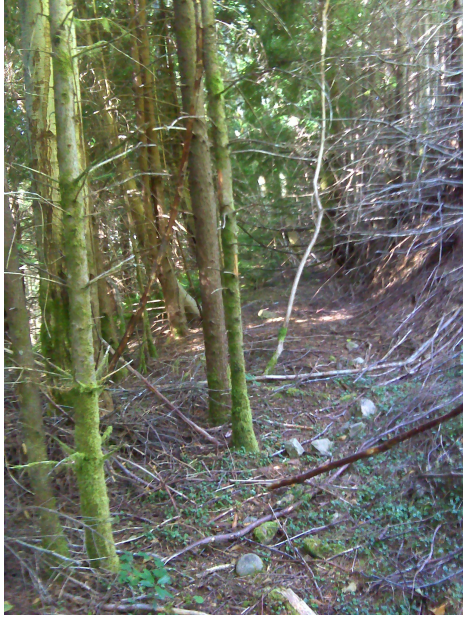
A33-2A N47 35.264 W124 01.955 Notes: steep slope; homogenous forest (dark, thick), tension cracks in the road. Road is sluffing Direction: 245°
